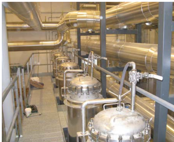
Figure 9: Picture with cartridge filters from geothermal loop in Sønderborg
