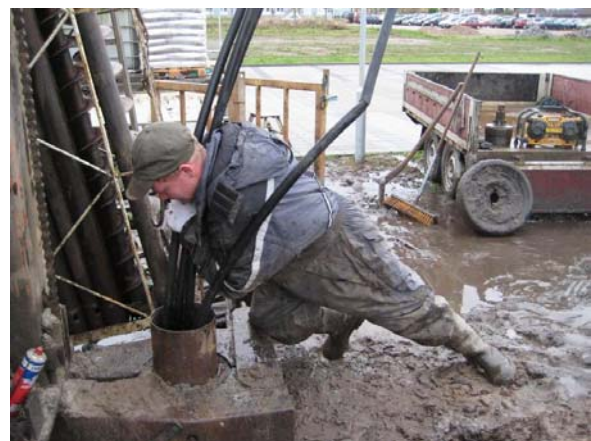
Figure 13: Installation of borehole heat exchanger at test site, photo Inga Sørensen VIA UC.
