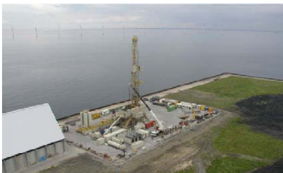
Figure 8: Geothermal plant in Copenhagen
